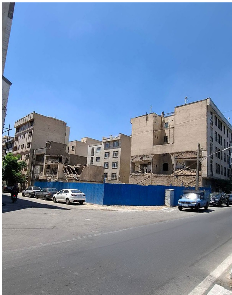
The use of high-powered munitions caused damage to adjacent locations in addition to destroying the primary target. ©HRA
