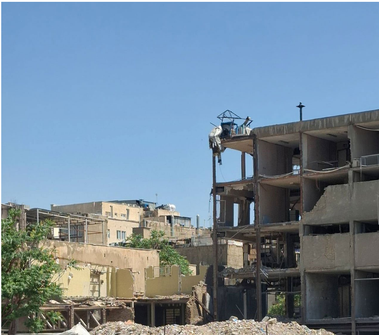
A residential building has been destroyed as a result of airstrikes.
