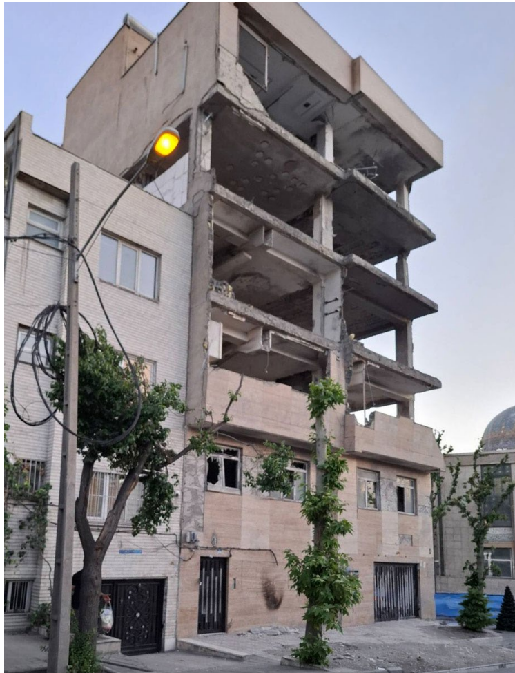
A residential building that was targeted in airstrikes ©HRA
